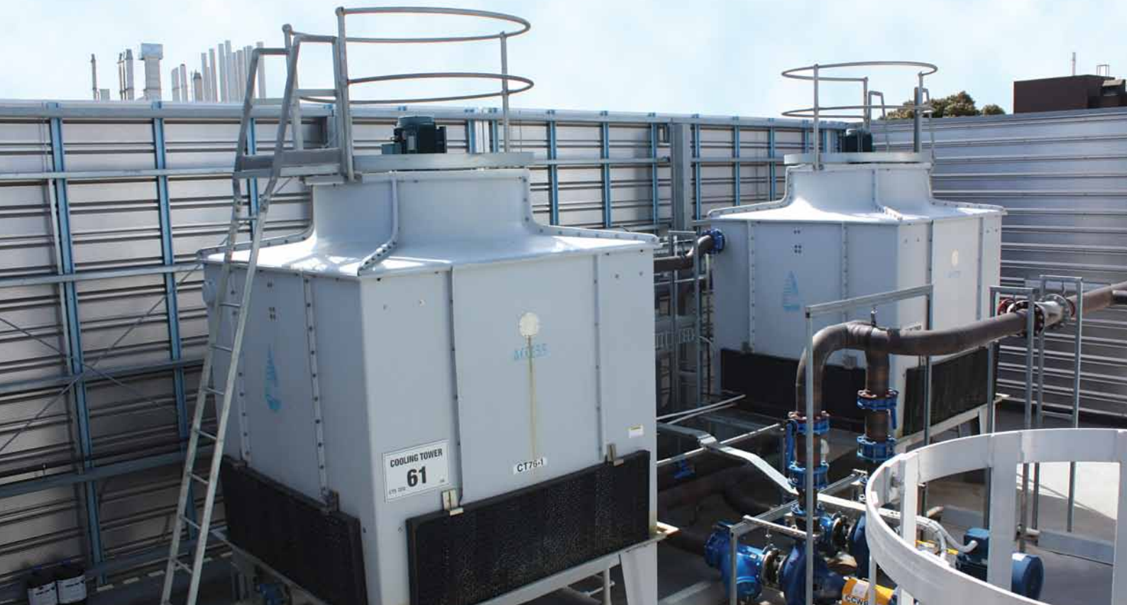
Cooling tower setup at Monash University
