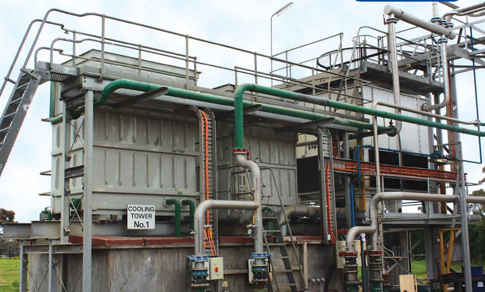
Cooling tower setup at Cryovac Rigid Packaging, Tullamarine
