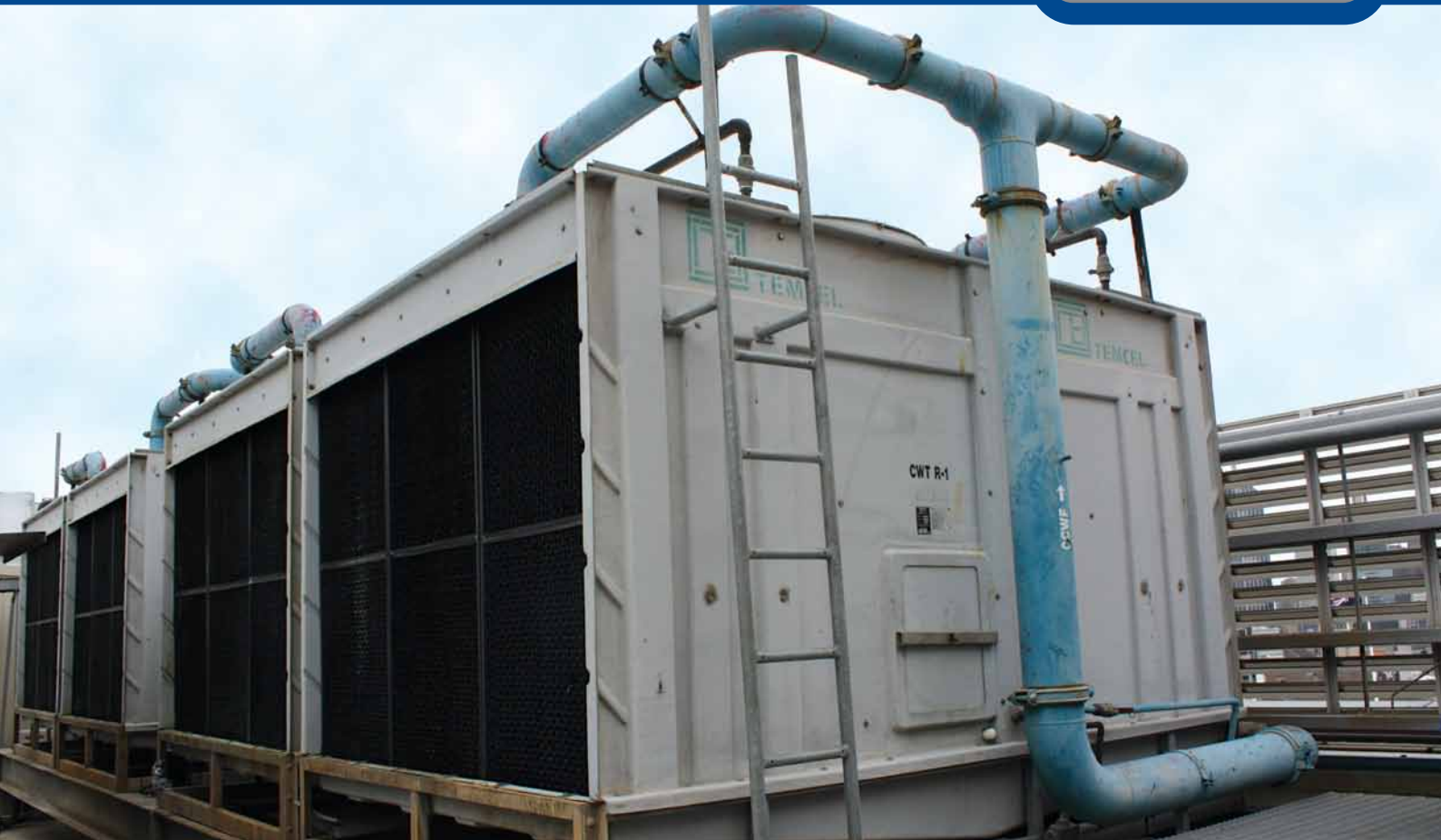
Cooling tower setup at Royal Melbourne Hospital, Victoria.
